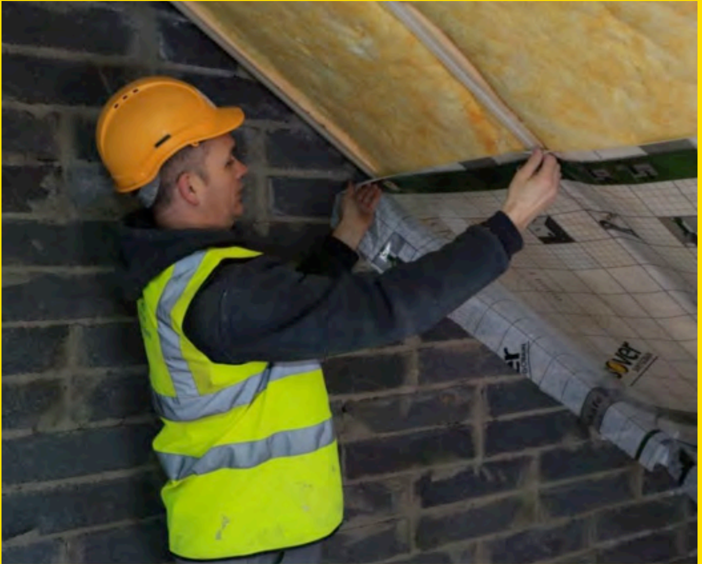
Vapour Barrier applied carefully to underside of Rafters in attic to prevent moisture getting in. This also requires a ventilation space above the insulation to avoid interstitial condensation. Image courtesy of Isover, Saint Gobain
