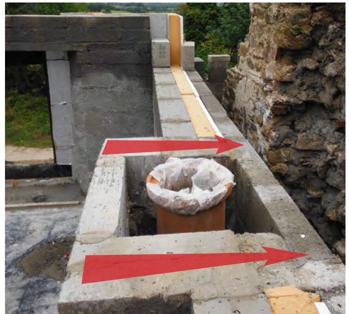
The arrows in this photograph show where a thermal bridge has been formed by the chimney structure which passes right through the insulation layer. Image courtesy of Gavin O'Shea
