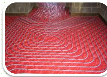
Floor, radiator, and Convector heating systems
