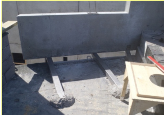
Figure 3.5. On the one hand, energy-saving wall solutions are being sought while at the same time thermal bridges and other energy-losing solutions are being designed.
