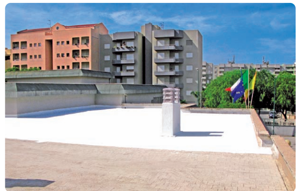
Figure 14. View of the roof with a partial application of the cool roof paint
