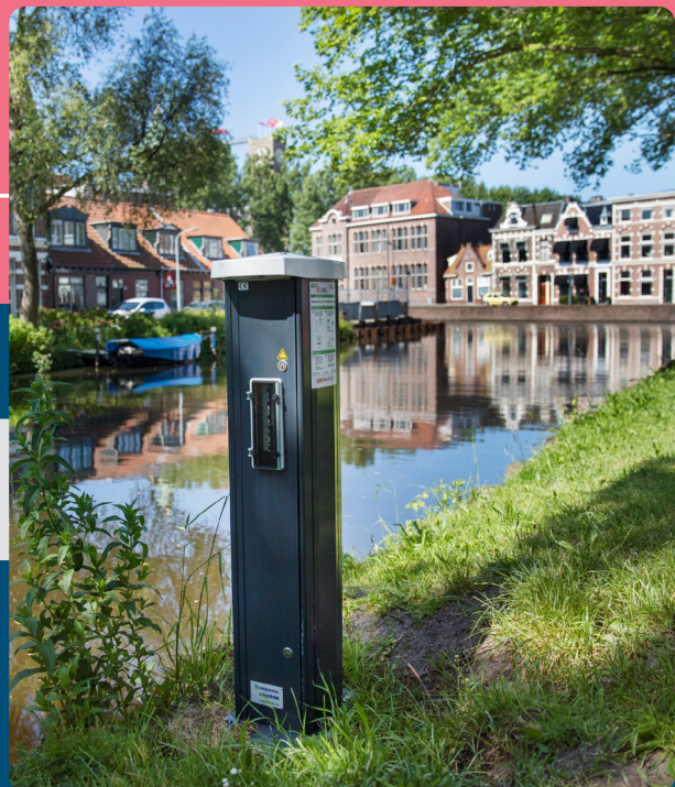
Boat charging stations procured through circular criteria. Image: Gemeente Haarlem
