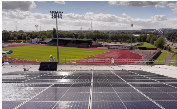
2,000 solar panels are installed on the Geraint Thomas National Velodrome in Newport – © Mike Harrison
