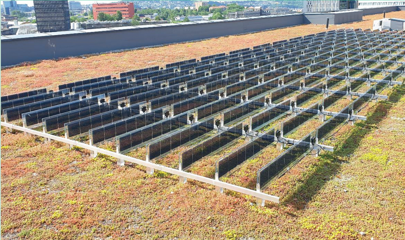
Pilot installation of vertical bifacial solar panels on green rooftop in Oslo.
