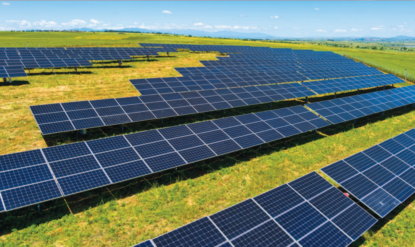
PV park in Greece.
