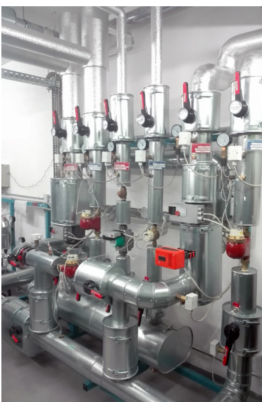
Photo 13. Heating manifold for radiators and ventilation with flow meters Source: Polish Institute of Urban and Regional Development
