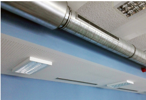
Photo 11. Extraction and supply of air from/to a room Source: Polish Institute of Urban and Regional Development.
