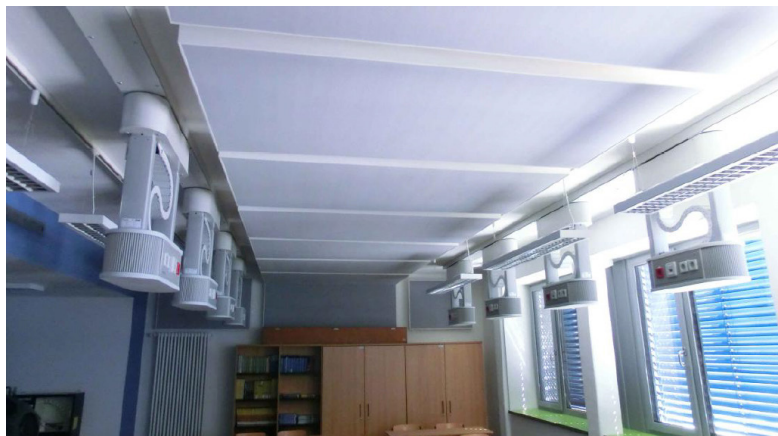
Photo 14. Physics classroom with soundproof panels in the ceiling and retractable media Source: Sanierung Max – Steenbeck – Gymnasium Cottbus. Schlussbericht, Cottbus, September 2015: p. 32; https://web.archive.org/web/20180315134705/https://projektinfos.energiwende-bauen.de/projekt/energetische-sanierung-einer-plattenbau-typenschule .
