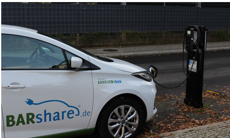
Photo 4. Electric charging station capable of feeding electricity back into the municipal grid
