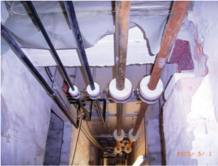
Photo 9. Installing a water and central heating system prior to insulation; the photograph shows a special fastening system using hard foam insulation that eliminates the risk of gaps forming and the insulation layer thinning Source: Polish Energy Conservation Foundation.
